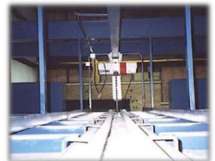
Overhead Material Handling
